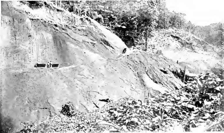
A SLIDE IN A CUT, DUE TO HEAVY RAINS.
